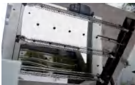
3 Heating tubes Drying system
